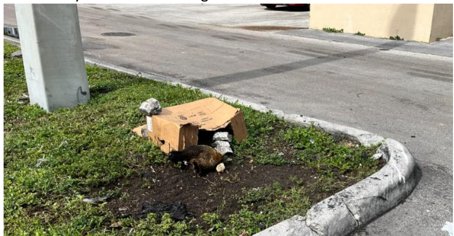
FIGURE 3: LANDSCAPE ISLAND WITH BROKEN CURBS, EXPOSED SOILS, AND A CARBOARD BOX PROVIDING TEMPORARY SHELTER TO SOME WILD
