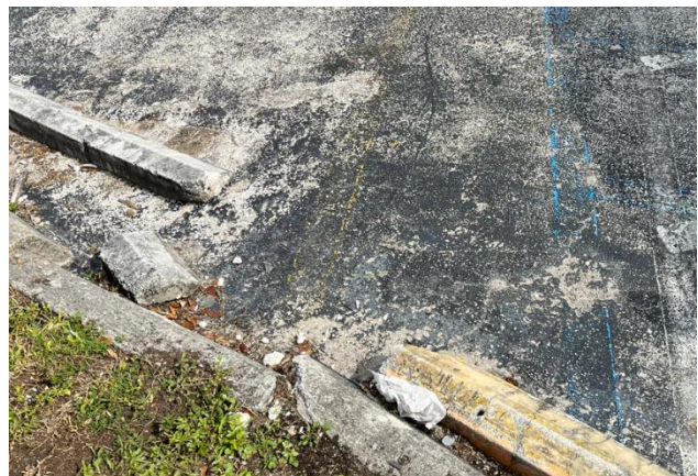
FIGURE 5: BROKEN CURB, BROKEN WHEEL STOP, AND ANOTHER MISPLACED WHEEL STOP
